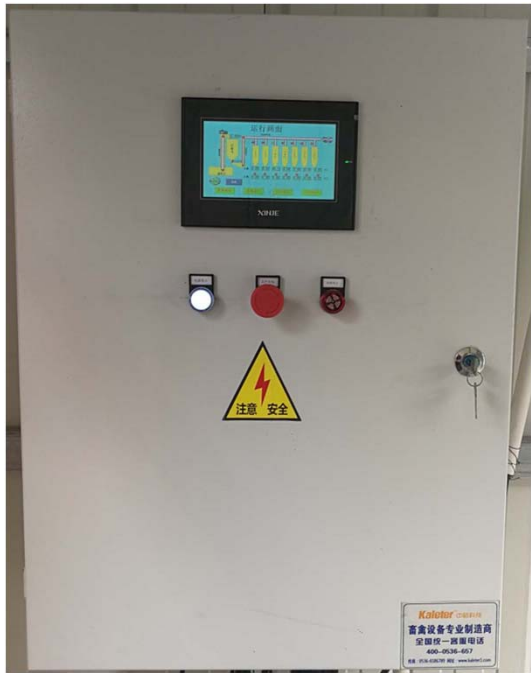
House weighing control panel
